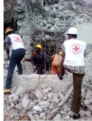
NRCS Volunteers and other response partners on a search and rescue mission in a collapsed building site
